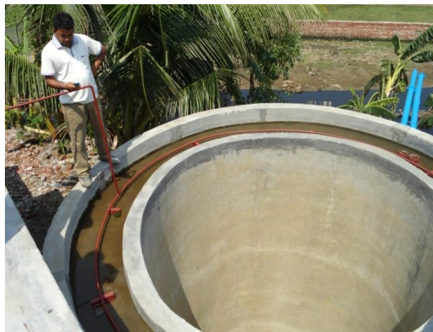
Secondary Clarifier with Post Aeration System
